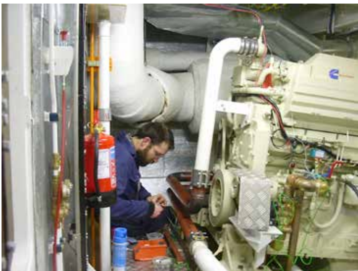
Exhaust ducting vibration measurement in an engine room
